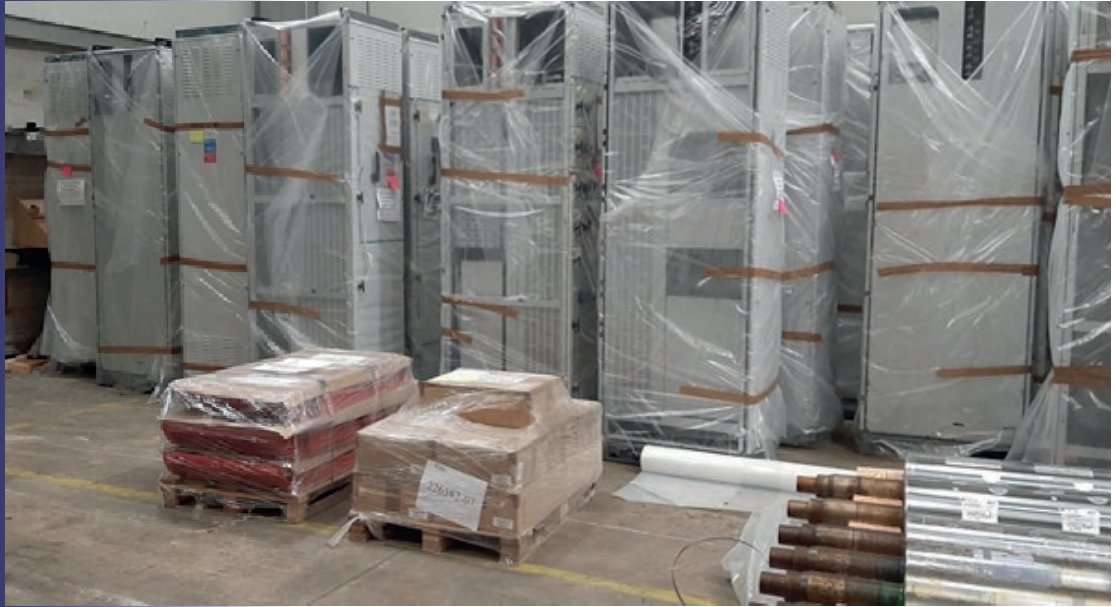
P98 Level 2 Switchboards
