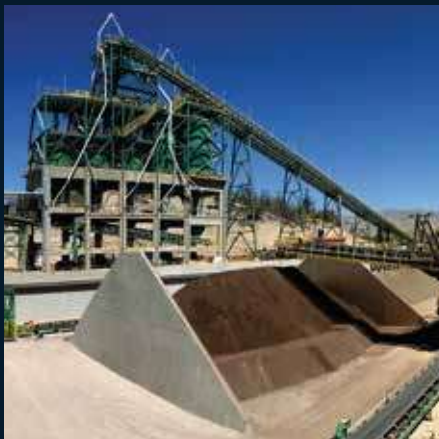
Claudius Peters Limestone Bridge Reclaimer, North Africa
