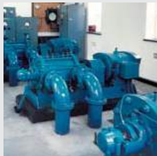
Potable Water Pump.
