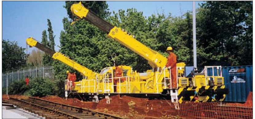
Twin jib panel and sleeper cranes laying dual track sleepers. London Underground
