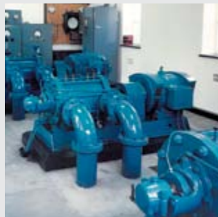
Potable Water Pump.
